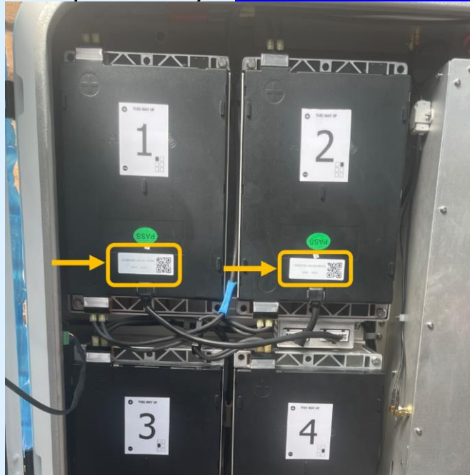
Figure 9 – Installed ElektroBank 14 battery modules showing location of serial number QR Code
